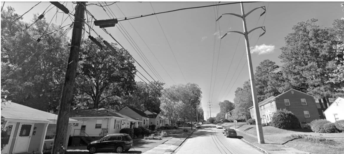
Figure 2: Wood and metal OHLs of different voltages above a residential street in Durham, North Carolina.
